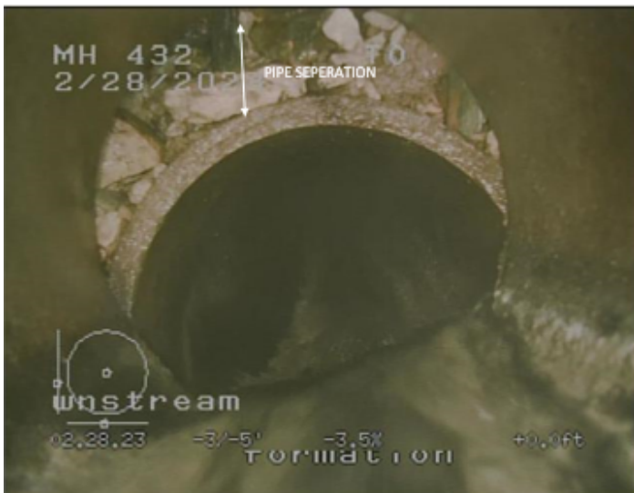
Photo 3. Camera view inside an active sewer pipe in East Whiteland, Chester County shows pipeline break which allows raw sewage to enter the environment.
